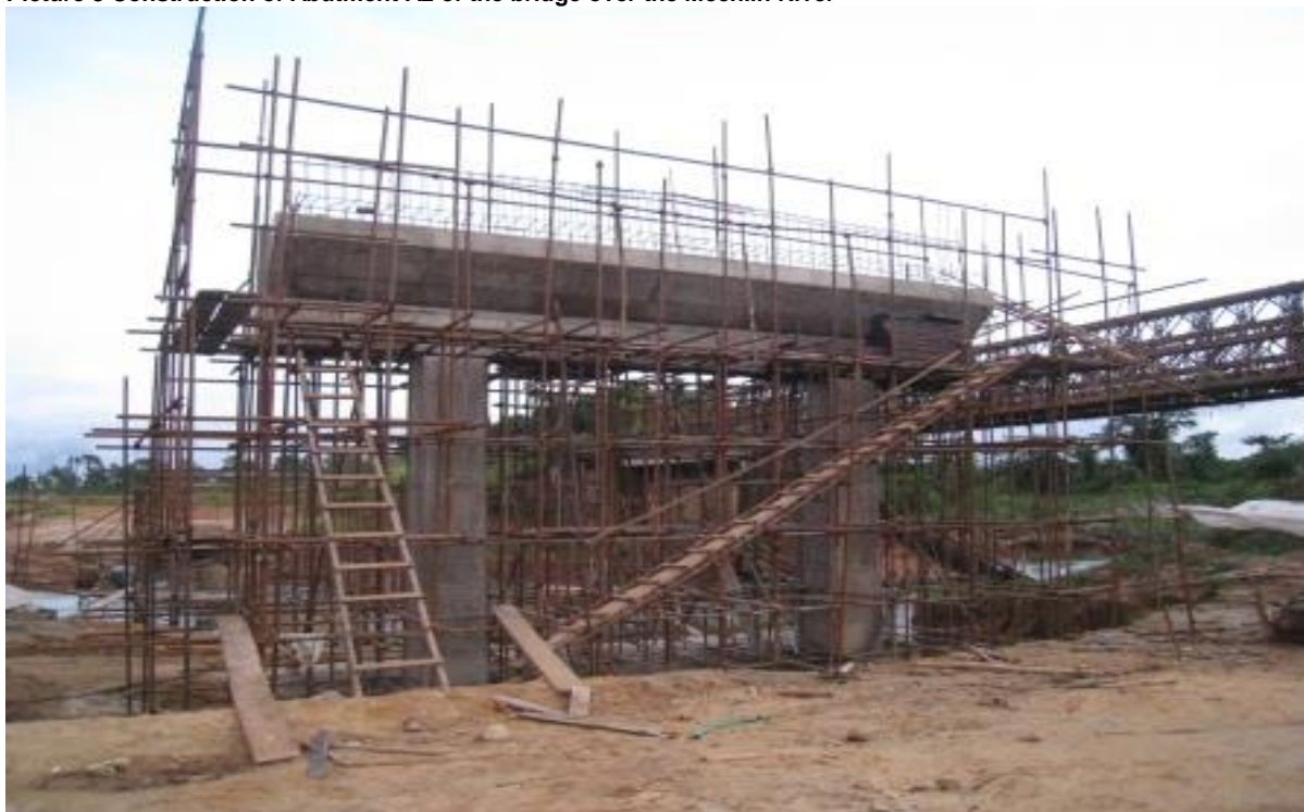
Picture 3 Construction of Abutment A2 of the bridge over the Mechlin River
