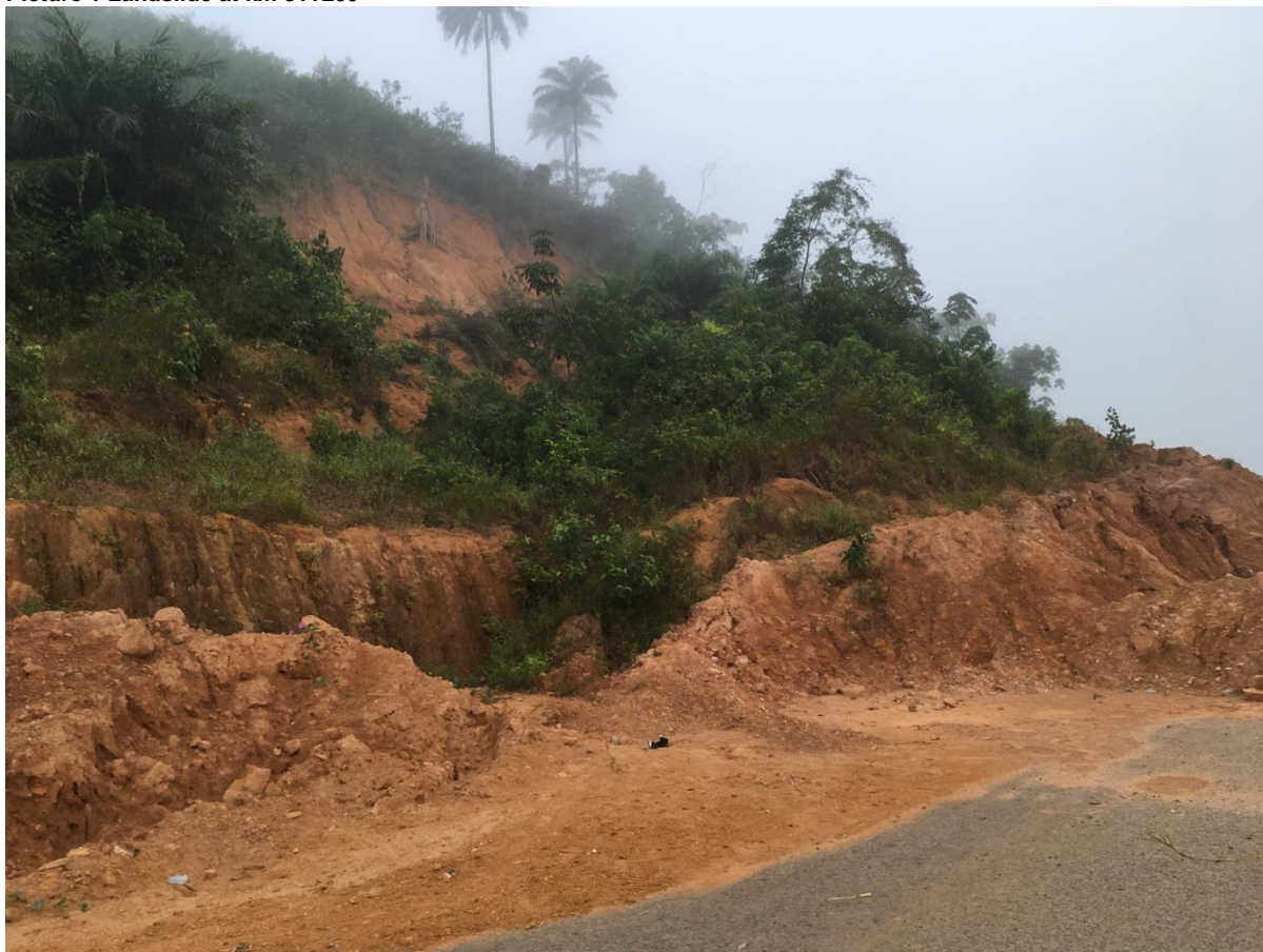
Picture 1 Landslide at km 31+200
