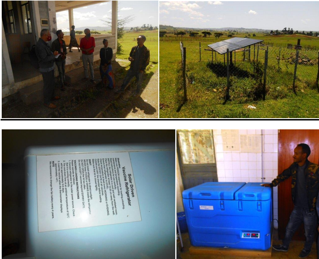
Picture (set) 3: The MTE team interviewing the Health Center staff in Jarso (top-left), the 1,200Wp Solar PV array at the Jarso Health Center (top-right); the refrigerators in use at the Jarso Health Center (bottom-left and bottom-right)
