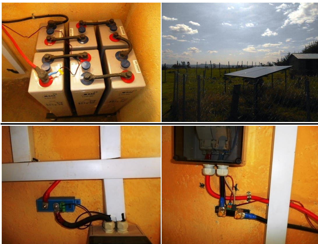
Picture (set) 4: The 12V battery pack (top-left) and the 600Wp solar PV array at the Dumburii Health Post (top-right) and some of the connections constituting the installation at the Health Post (bottom-left and bottom-right).
