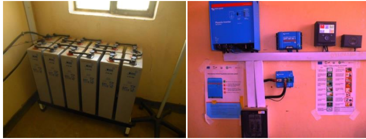
Picture 2: Battery connected in series and the power electronics installed at one of the larger capacity system sites visited by the team
