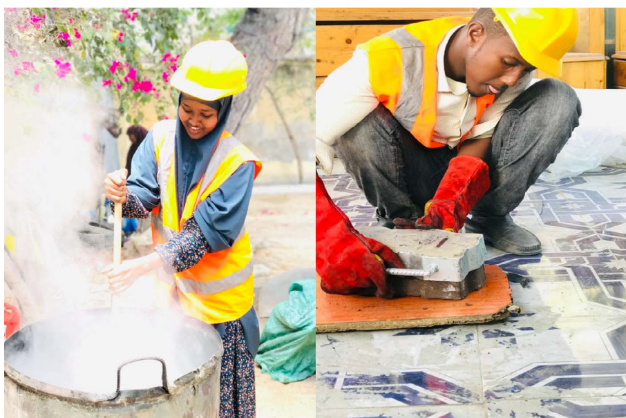
BRIDGES' road construction trainees from Halye Barrise TVET Centre do practical field work as part of a construction project in Mogadishu, Somalia.
