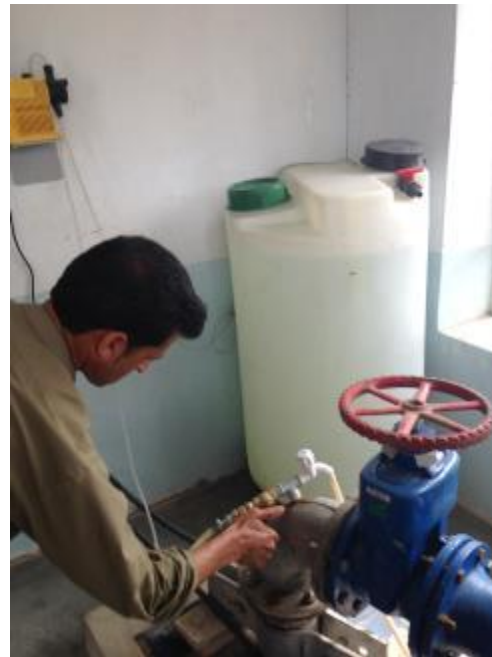
Chlorination at the pump unit
