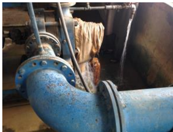
The functioning pump in the middle (note the leakage under the cloth, estimated at 50% of the capacity)
