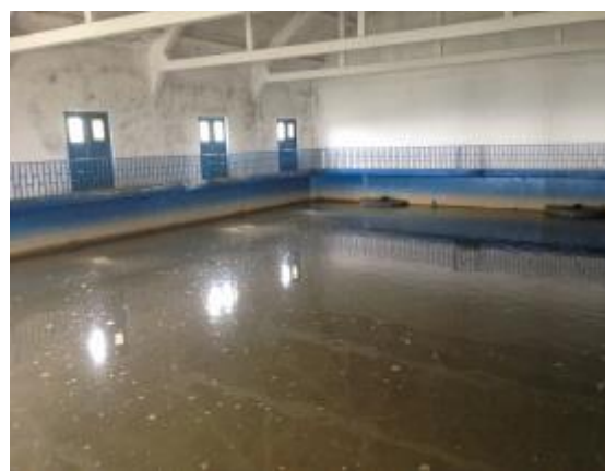
The sand filter of the treatment plant
