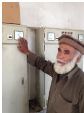
The pump house and electrical panels
