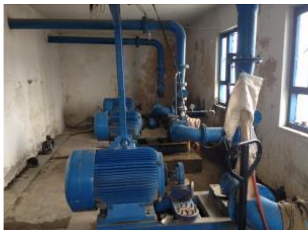
The pump house at the canal (note that the first and last pumps are not connected)
