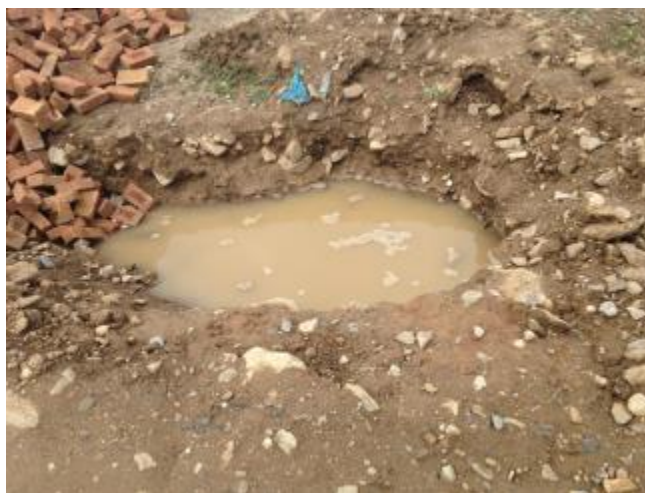
Leakage in upstream distribution pipe
