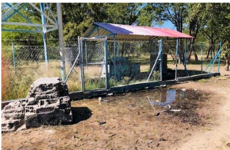
Photo 12: Epango, potable water flooded access near cattle infrastructure
