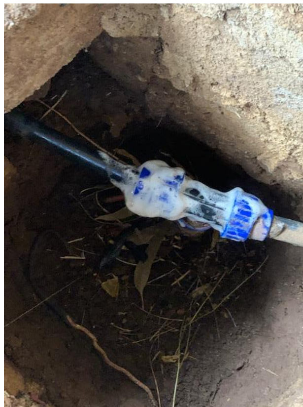
Exhibit 8. Gas leakage uncovered during the technical evaluation mission Banja Woreda, Awi Zone, Amhara Region
