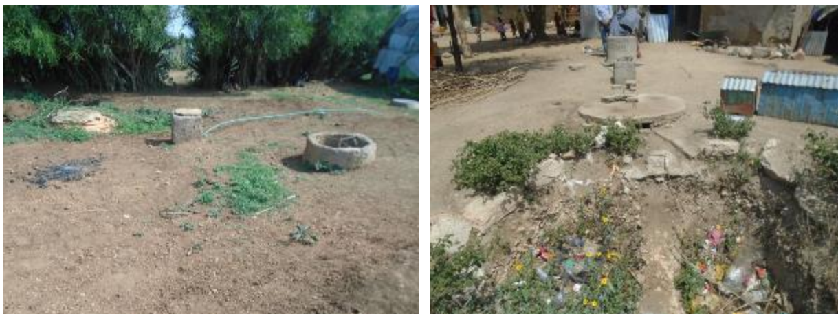
Figure 91 - Exposed pipes (left) and flat outlet (right) of bio-digesters
