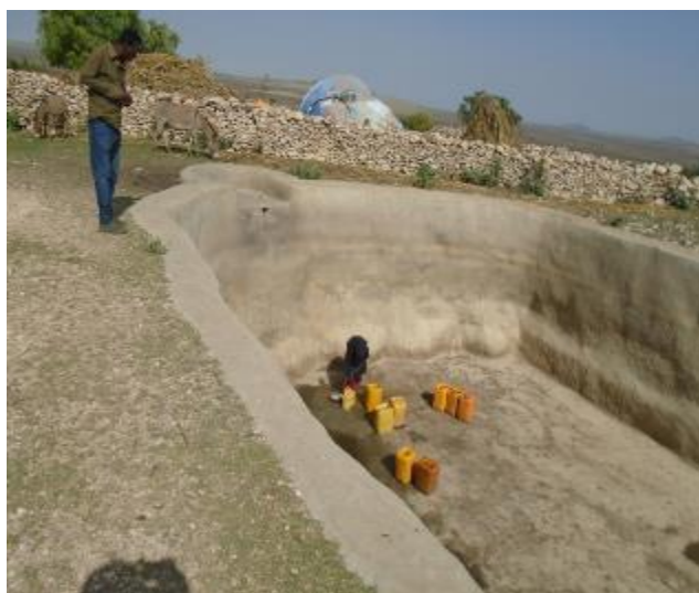
Figure 80 - Rainwater harvesting structure for dry season storage to be used for bio-digester in Owbarre Woreda
