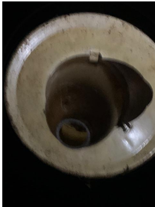
Exhibit 10. Broken lighting, Guangua and Banja Woredas, Awi Zone and Mechakel Woreda, East Gojjam Zone, Amhara Region Amhara Region
