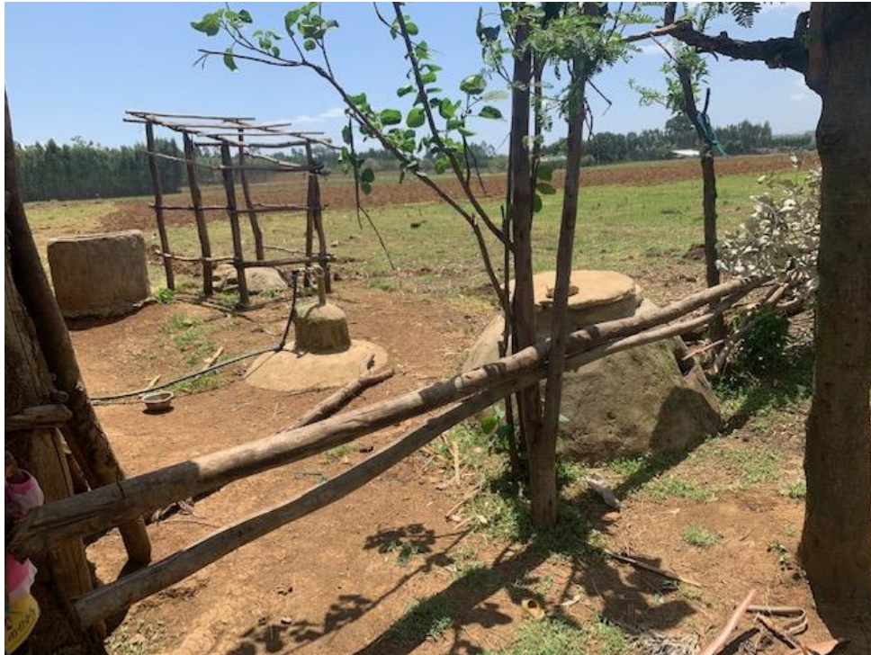
Exhibit 7. Unprotected Gas pipeline exposed to damage by animals and children, Dangla Woreda, Awi Zone Amhara Region.
