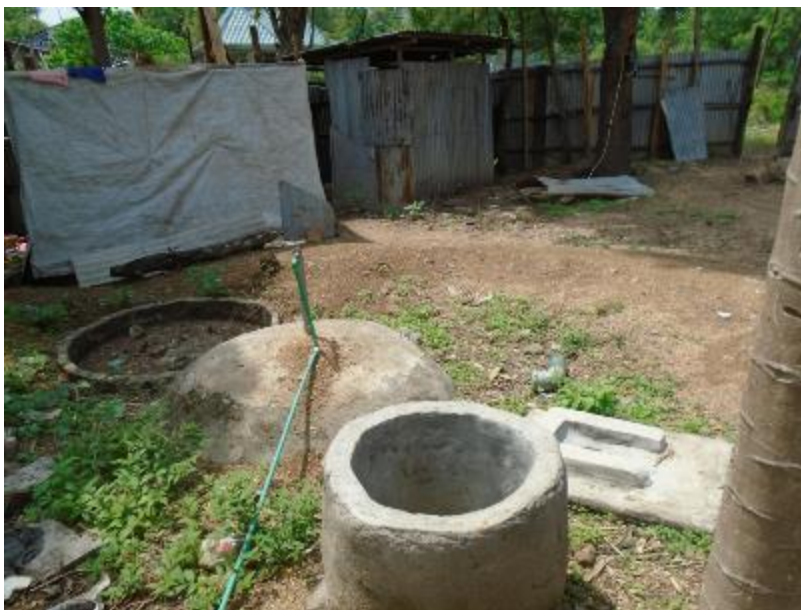
Figure 42 - Incomplete bio-digester under construction for over one year. (Gambella_ Anywaa_ Gambella Zuria_ Gambella Town_ GM AB 24_ Year 3_2020_ David Omo Okori)
