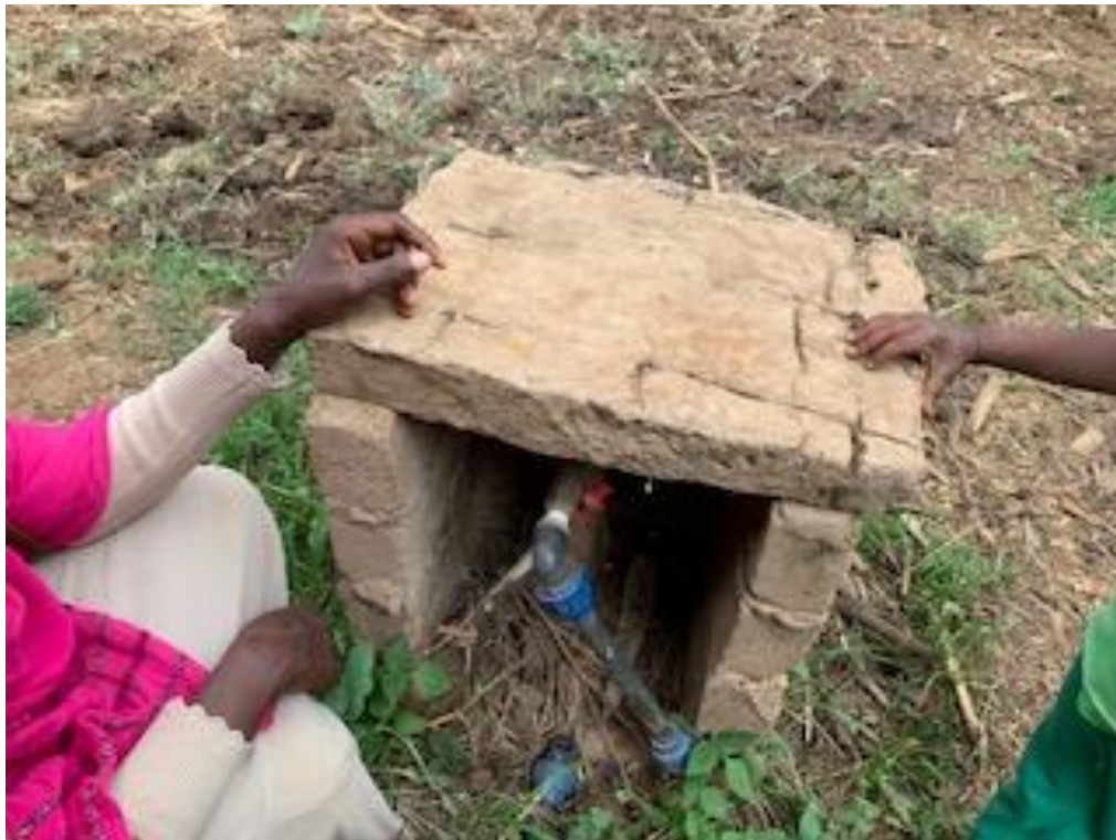
Exhibit 3. Broken pipeline, Gozamin Woreda, East Gojjam Zone Amhara region
