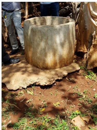
Figure 95 – Not properly covered dome affecting the stability of the inlet.
