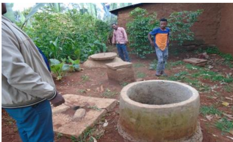
Figure 75 - Well-constructed bio-digesters with toilet connected but not used (SNNPR_ Wolayita_ Boloso sore_ Wurmuma_ Sn-hope-284_ Year 3_2019_ Dawit Gua)
