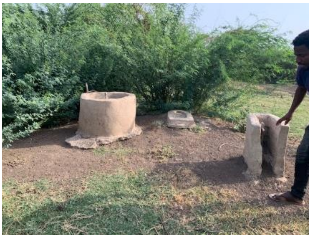
Exhibit 6. Broken pipeline, Assayita Woreda, Zone 1, Afar Region
