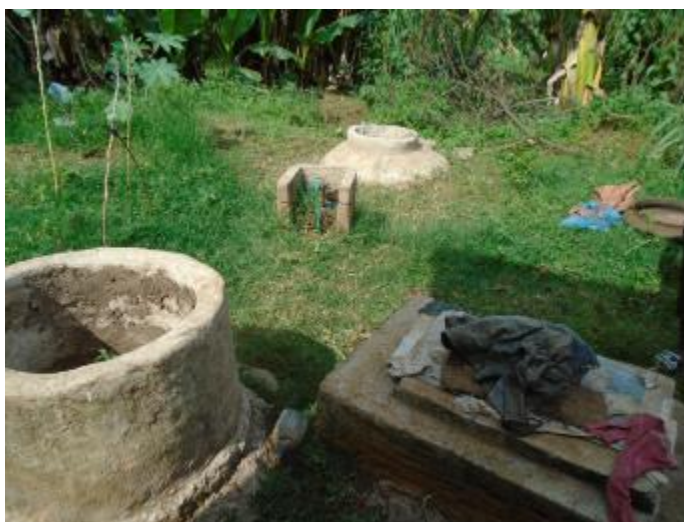
Figure 63 - Poor finishing in bio-digester, turret not covered and unutilised toilet (SNNPR_ Wolayita_ Boloso sore_ Arka 02_4940_ Year 3_ March,2020_ Dereje Wogaso)
