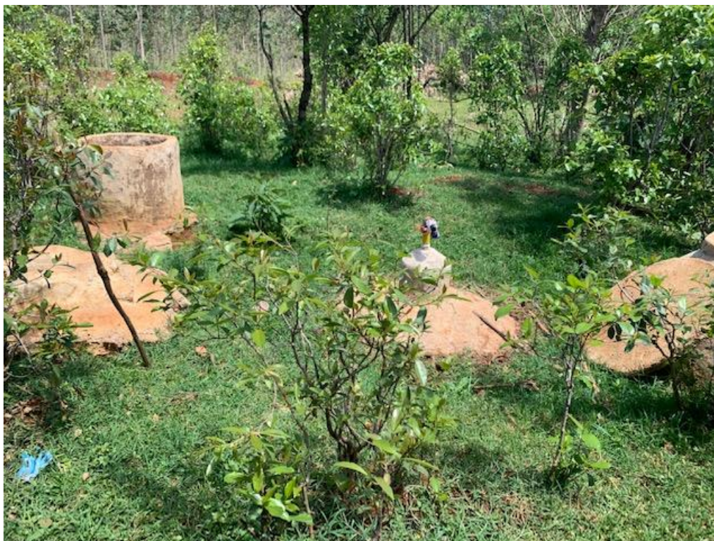
Exhibit 5. Broken pipe, Dangla Zurya, Awi Zone, Amhara region
