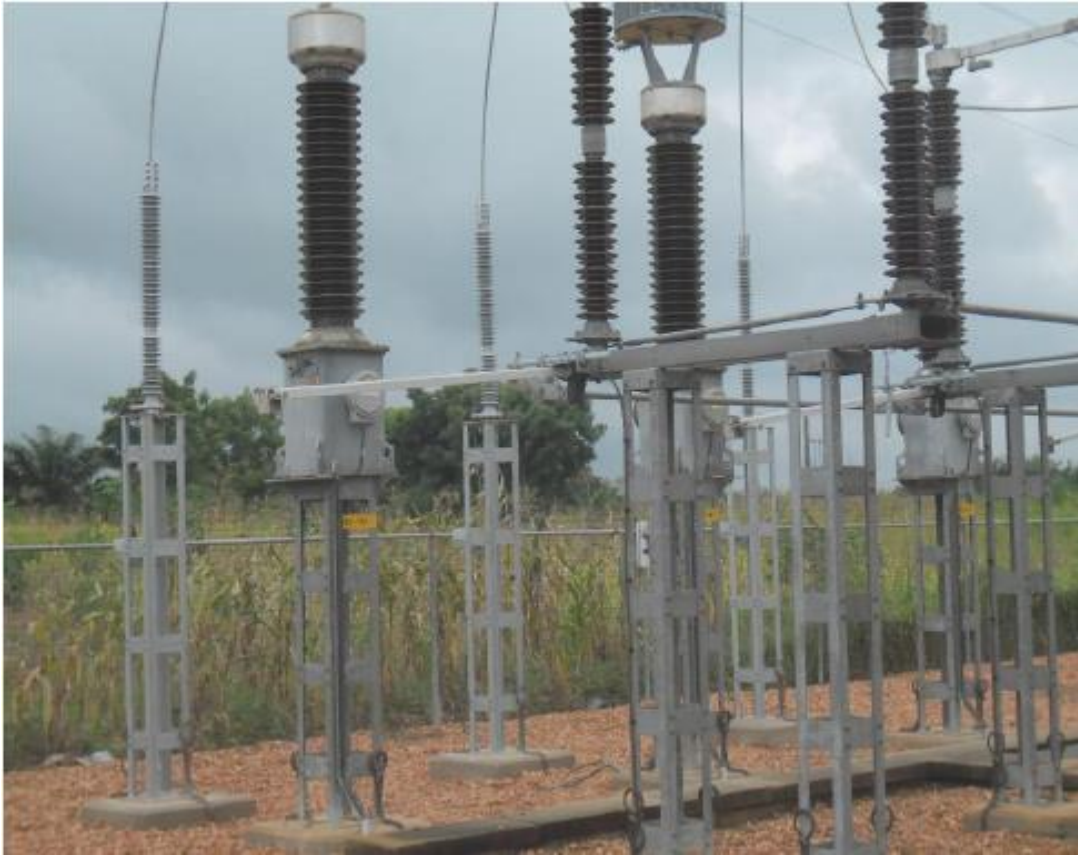
New Surge Arrestors in Vedoko (Benin) Substation installed by Benin and Togo Power Rehabilitation Project (LCO)
