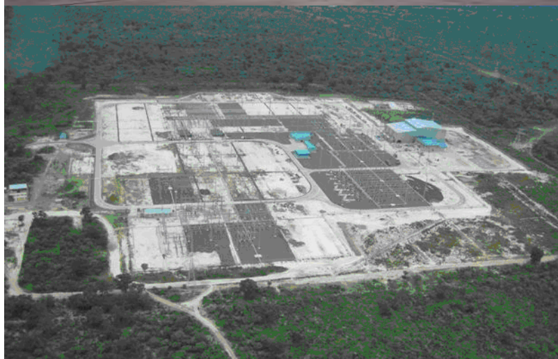
Rows of semiconductor units for converting current www.eu-africa-infrastructure-tf.net Gerus substation Source: ABB
