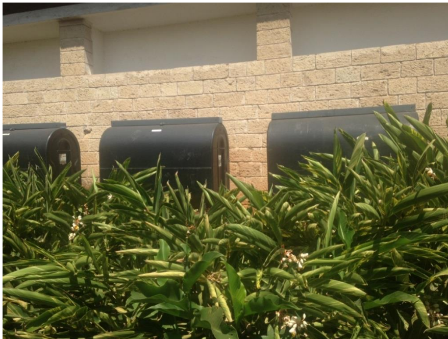
Figure A3: Photograph showing an array of stand-by diesel generators at Strathmore Business School whose use has been significantly reduced since installation of the solar PV modules
