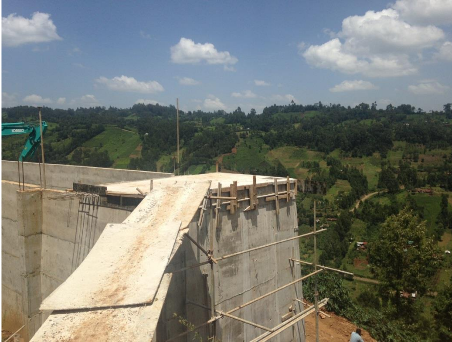
Figure C1: Photograph showing a section of the forebay under construction at KTDA's Gura small hydropower project in Nyeri
