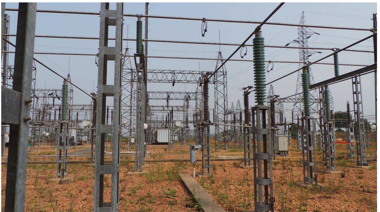
Aflao (Togo) 161 kV Substation Rehabilitated by Benin - Togo Power Rehabilitation Project (LCO component)
