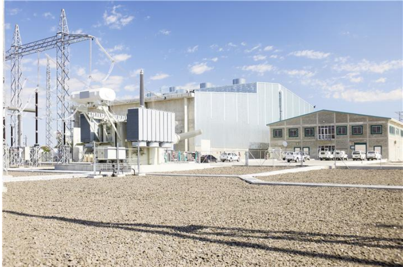
Gerus converter station Source ABB
