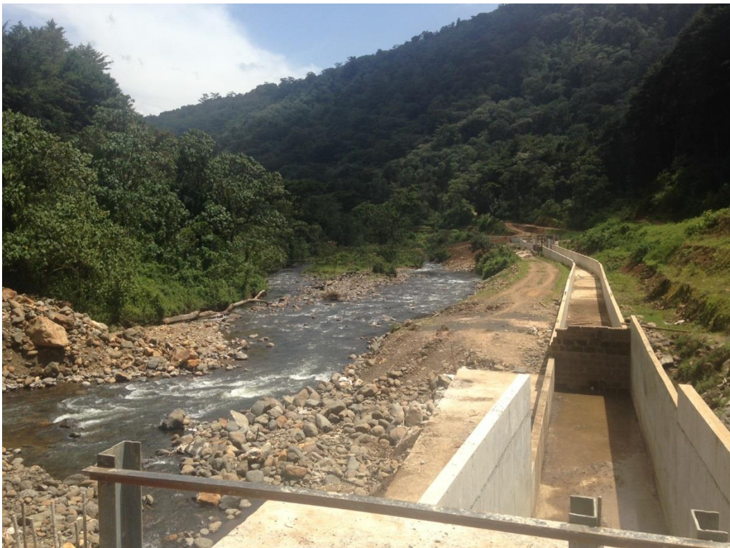
Figure C4: Downstream view of a section of the Gura Small hydropower project water canal
