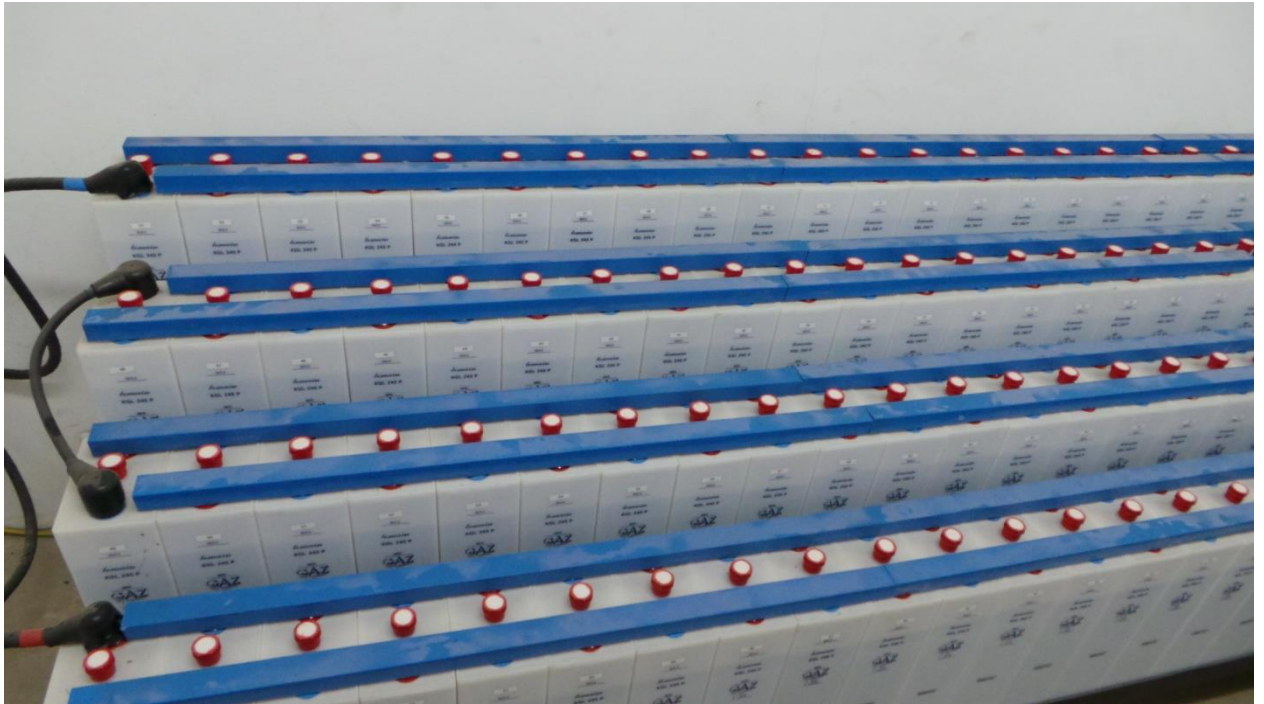
New 125 V Battery installed in Aflao (Togo) 161 kV Substation by Benin - Togo Power Rehabilitation Project (LCO component)
