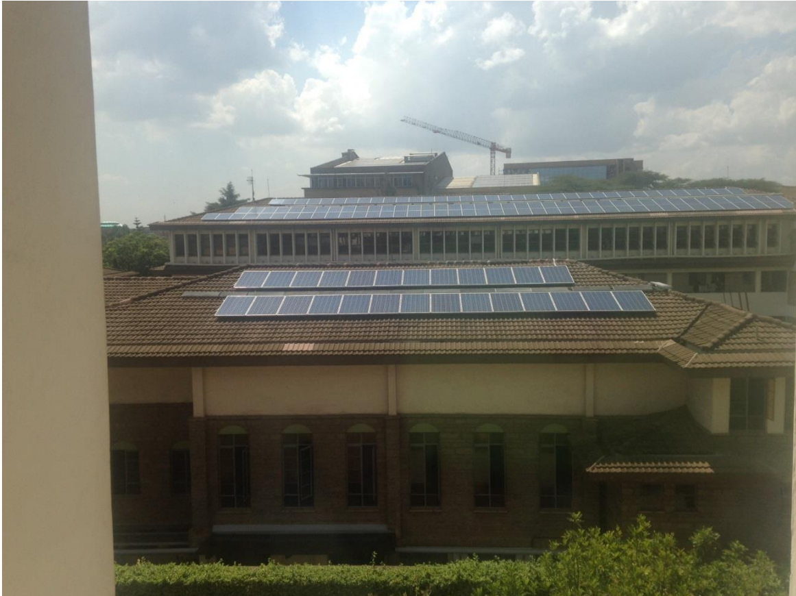
Figure A1: Photo showing a section of the 600KW roof-mounted solar PV panels at Strathmore Business School
