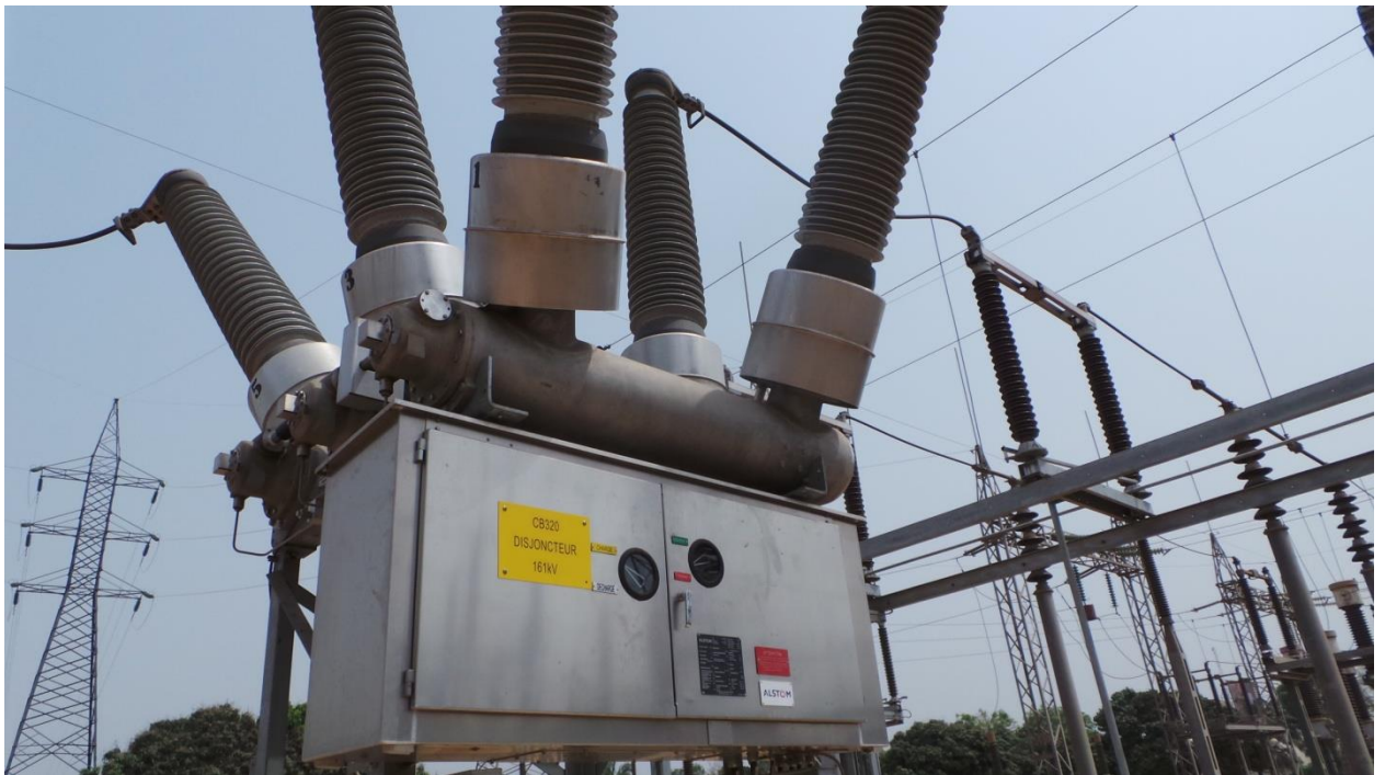
New 161 kV Circuit Breaker in Aflao (Togo) Substation installed by Benin - Togo Power Rehabilitation Project (LCO component)
