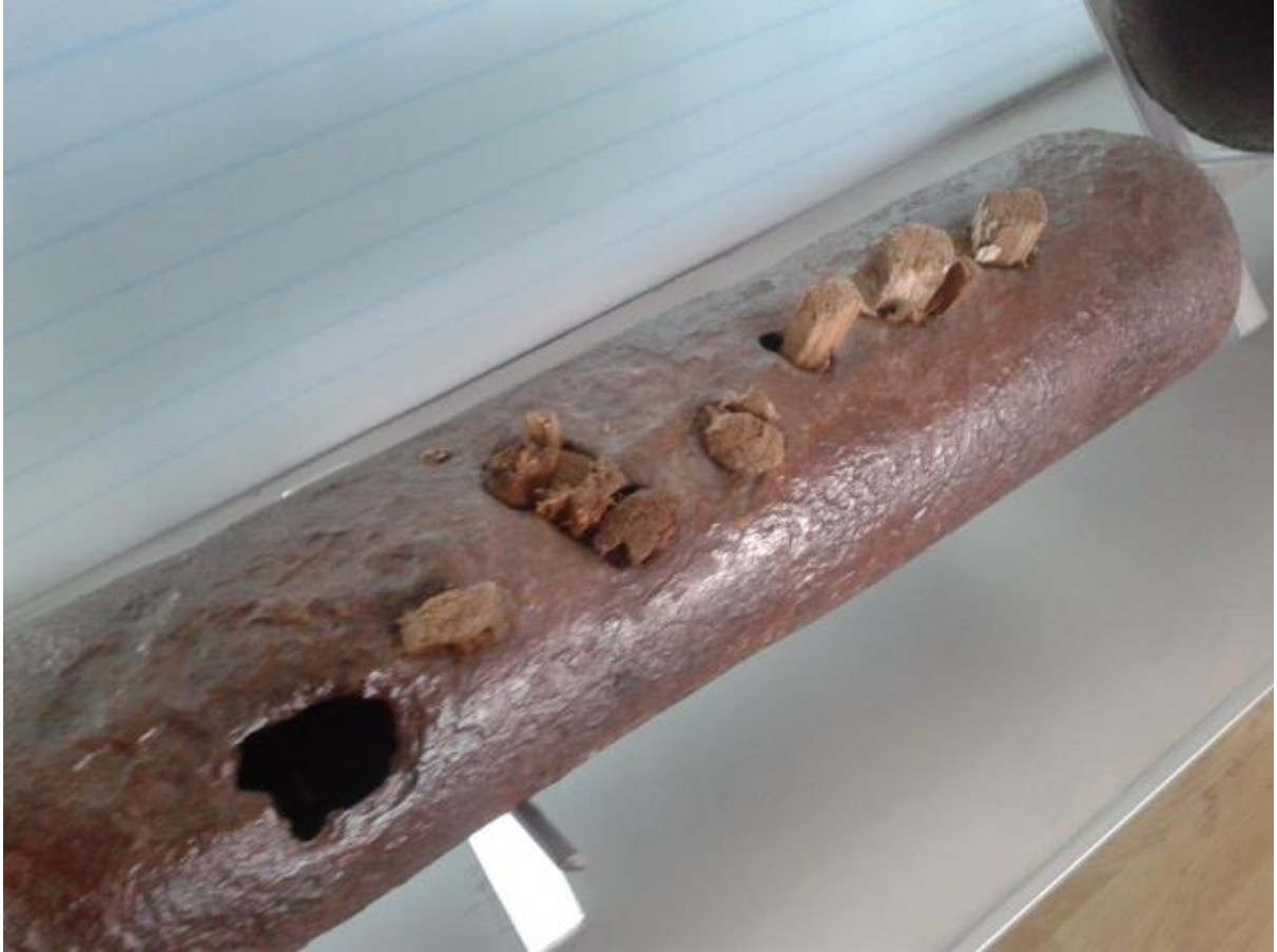
Fig 6 Traditional leakage control (the Armenian Small Municipalities Project used more modern technology)
