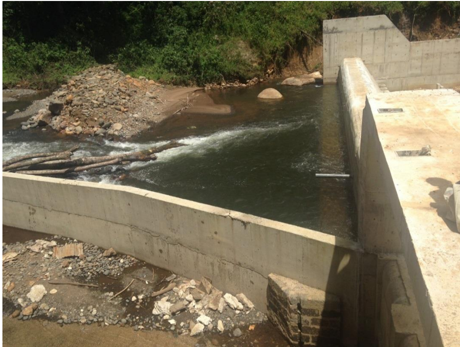
Figure C3: Intake channel showing gate chambers at Gura SHP project
