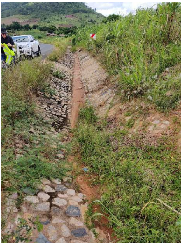
Ditch needs routine maintenance
