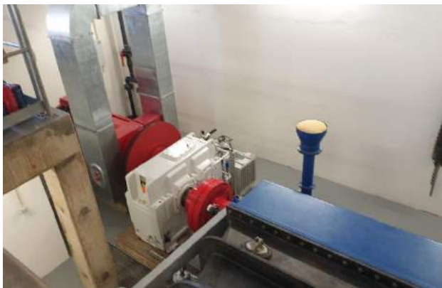
View inside the power station
