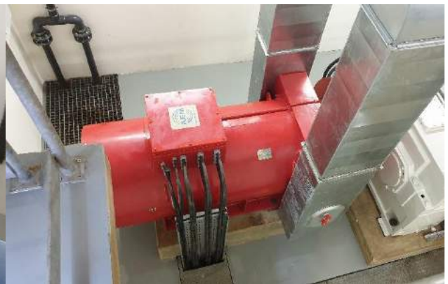
The power generation unit
