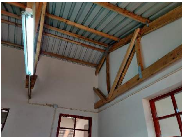
Inside view of the school. Note lighting powered by photo-voltaic cells
