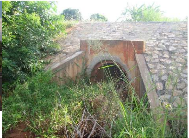
Routine maintenance required. Note good erosion protection around the headwall
