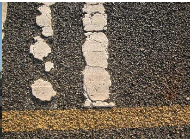
Rumble strips warn of speed limits, but these may need to be repaired before final handing over
